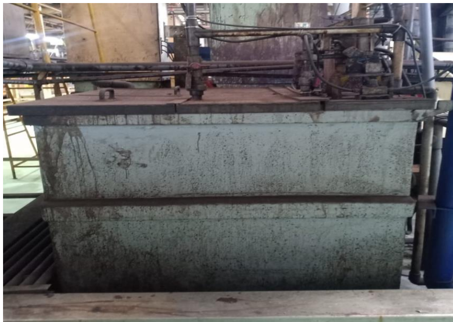
Gambar 5. Alat Mixing Chemical Cr 03
