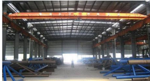
Figure 2 Overhead crane hoist to lift the cut plate to the assembly line.
